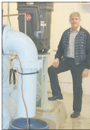
Courtesy City of Pendleton Bob Patterson, public works director in Pendleton, Ore., stands next to Aquifer Storage and Recovery Well No. 4. The well head and the 250 horsepower pump motor are next to him.
