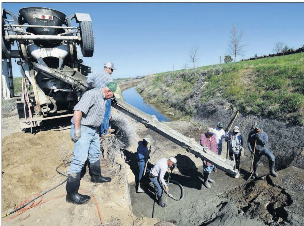
Workers with the Stanfield Irrigation District work on patching a ruptured spillway April 7 in one of their irrigation canals near Echo, Ore.
