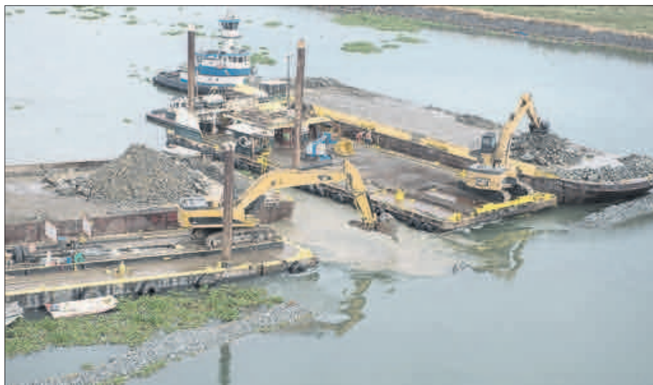
Crews remove a temporary rock barrier from the Sacramento-San Joaquin River Delta south of Sacramento in October. State officials say the March storms eliminated the need to reinstall the barrier, which was to keep saltwater from intruding in the drought-depleted Delta.
