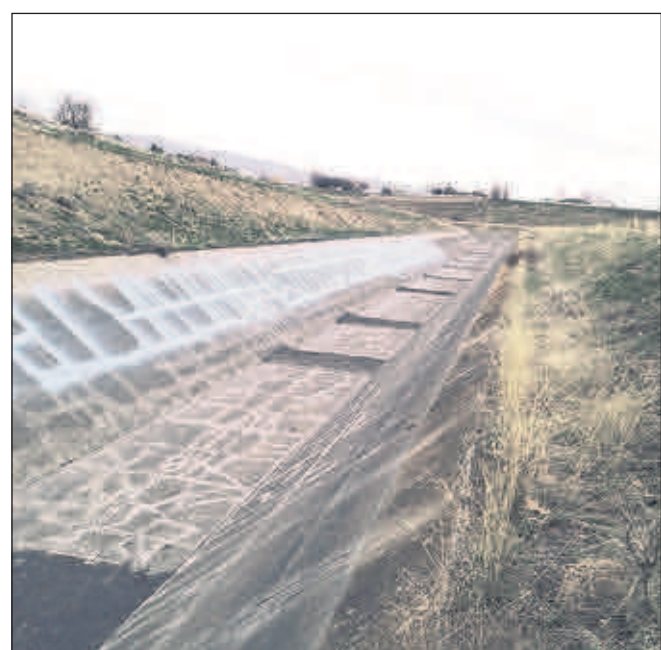
Courtesy/Roza Irrigation District Sealed cracks are on the sidewall and sandblasted cracks are ready for sealing on the bottom of the Roza Irrigation District canal
