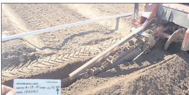
Courtesy Kinder Morgan Centerline Ag Services accidentally hit a pipeline transporting diesel and gasoline in late September near Aurora, Ore. The trench was being dug for irrigation equipment in preparation for blueberry planting.
