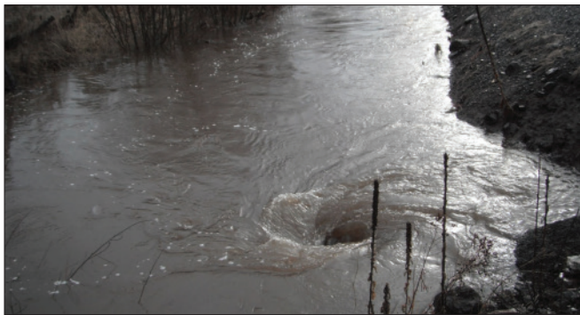
The inlet of the pipe at the confluence of Whiskey Creek and the Grande Ronde River is barely able to pass water on June 30, 2014, as it swirls into a vortex.
