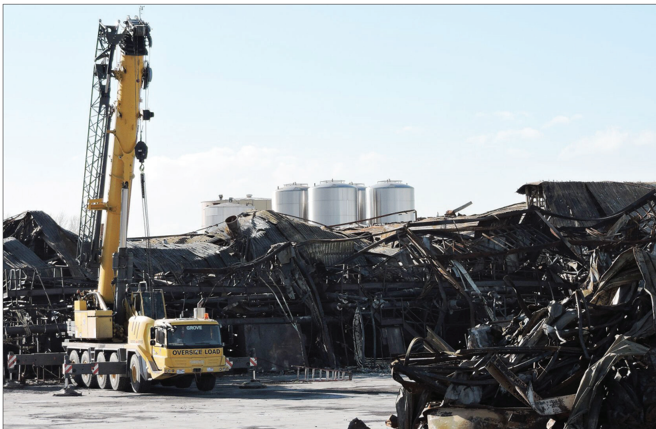
Equipment is in place to remove sections of debris from the destroyed Shearer's Foods plant in Hermiston on Monday, April 4, 2022.
