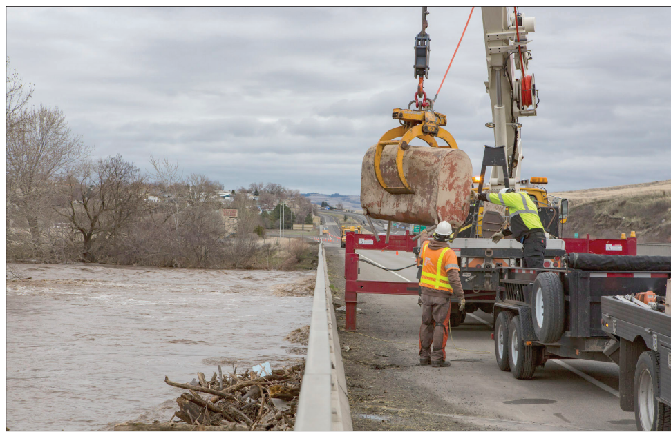
Above, Oregon Department of Transportation work crews remove debris that washed against the I-84 bridge over the Umatilla River in Pendleton on Friday, Feb. 7, 2020. Below, Chantal Fuller watches as water floods her home in Thorn Hollow outside of Adams on Feb. 6, 2020.
