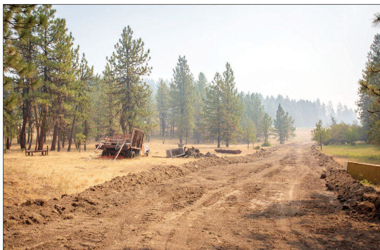
Ben Lonergan/East Oregonian A fire line, cut with a bulldozer, crosses the forest floor near Promise on Thursday, July 22, 2021, as fire crews work to stop the spread of the Elbow Creek Fire.
