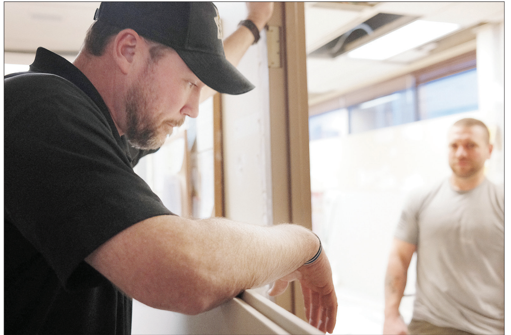
Union County Sheriff Cody Bowen leans over a piece of drywall in the sheriff's office on Friday, Feb. 19, 2021. One of Bowen's first acts as sheriff was to begin making renovations to the headquarters in La Grande, including tearing down a wall between deputies and supervisors.
