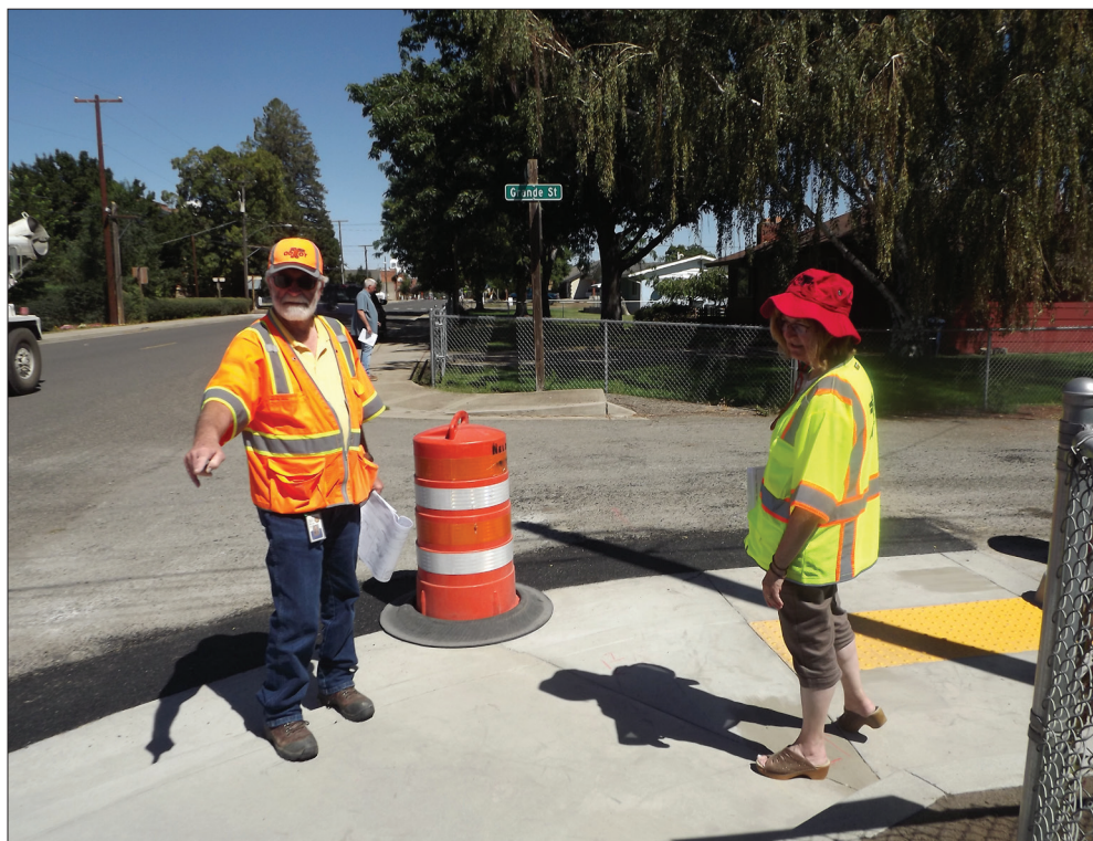
Staff photo by Dick Mason Howard Postovit and Leslie Hasse of the Oregon Department of Transportation examine a new curb ramp recently installed in Union.
