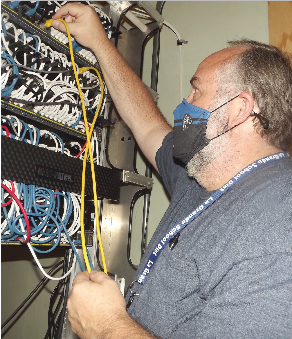
Staff photo by Dick Mason La Grande School District technology specialist Jeff Roberts examines one of the district's network closets Thursday, July 30, at Willow School, part of the district's computer technology infrastructure. It will receive heavy use from its students when school starts Aug. 31 because all of the district's students will take their classes via distance education.
