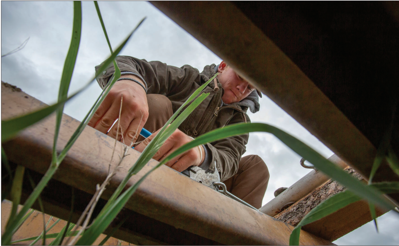
Spencer Shirtcliff tightens an eyebolt while installing an electric fence on a cattle guard Thursday morning while working as a ranch hand near North Powder.
