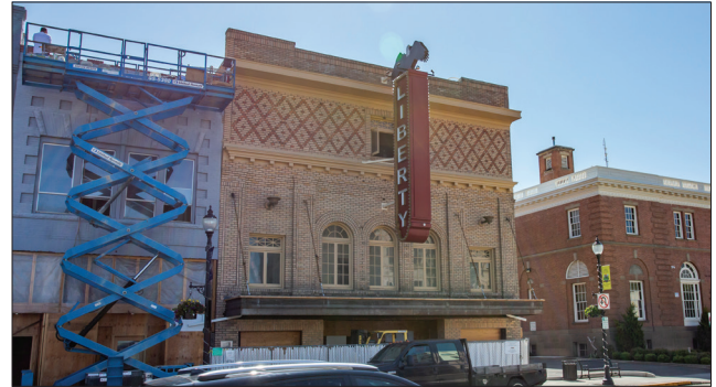
Restoration work continues on the Liberty Theatre in downtown La Grande in this May 7 photo. The foundation behind the restoration effort is seeking a $100,000 state grant for the next phase.
