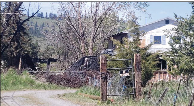
Staff photo by Sabrina Thompson An electric fire Saturday night on 12th Street in La Grande burned through this house.
