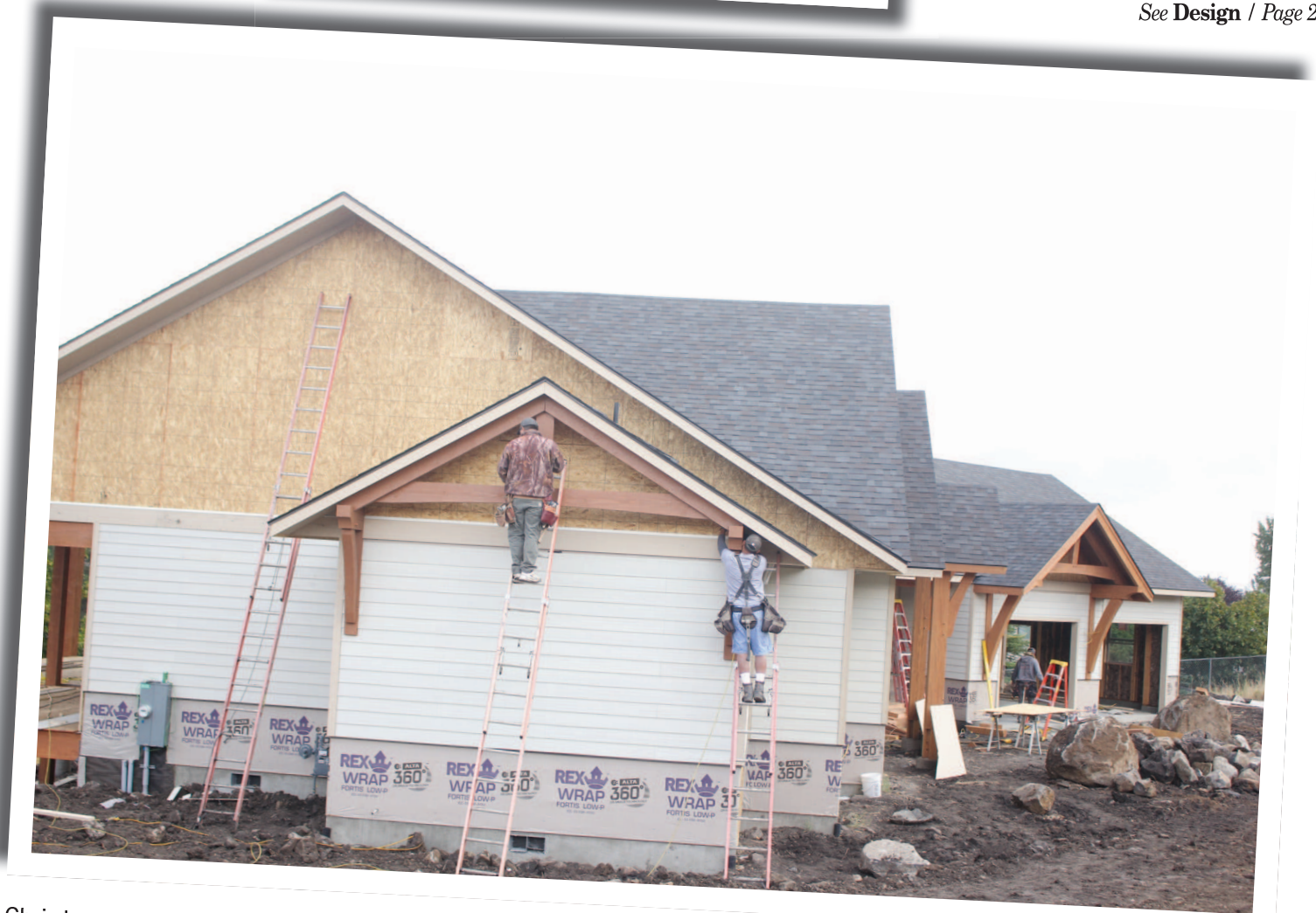
Chris Loman Construction employees are working on a new home that was designed by Ralph Edwards and engineered by Les Tipton near Birnie Park.
