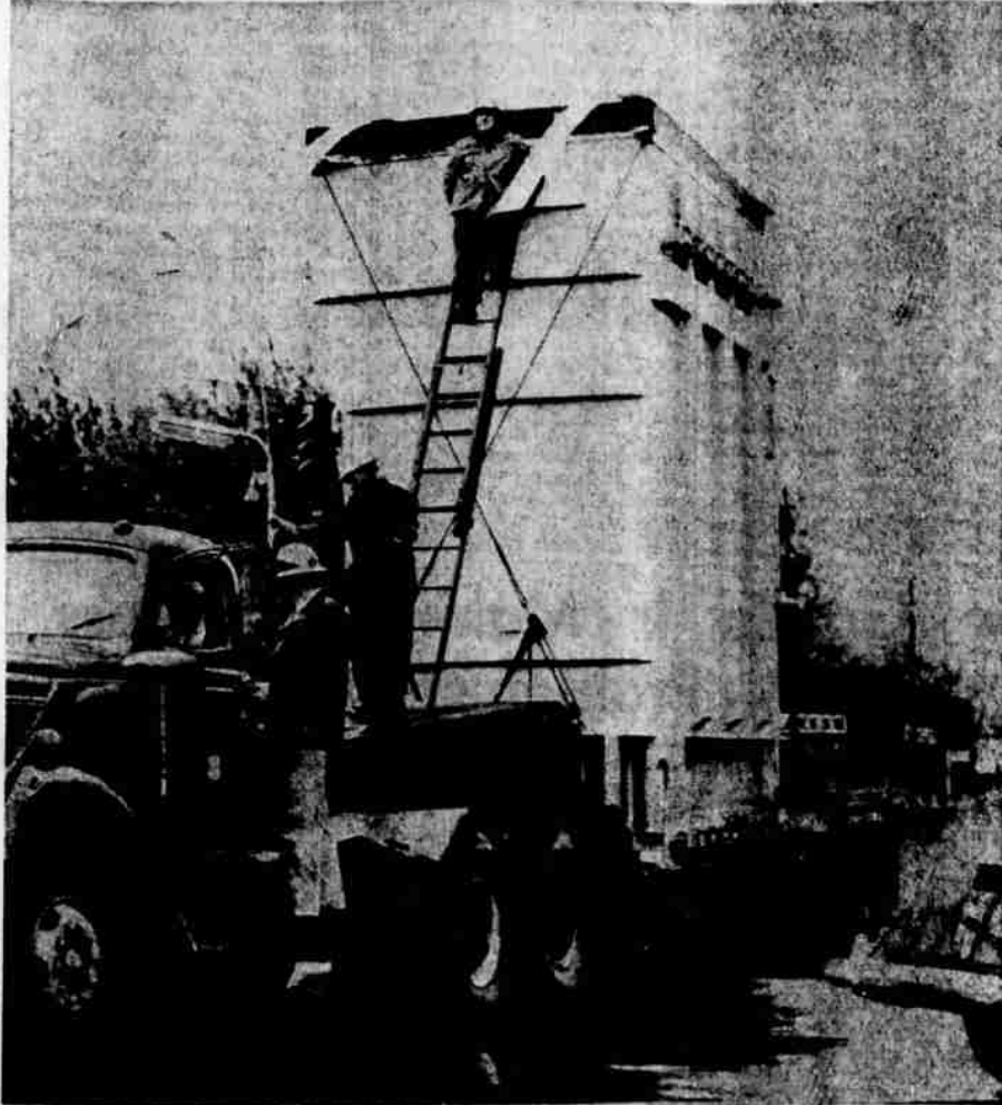
BIG TRANSFORMER —Bonneville Power crews slowed Fourth street traffic yesterday as they moved this 17½ ft. high transformer from the power substation south of La Grande to the UP tracks where it will be taken to McNary Dam by flatcar. The giant piece of equipment weighs 80 tons and has a capacity of 230,000 volts. The man on the top of the ladder used the two boards at the front to raise low power lines over the top of the transformer as the truck slowly moved down Fourth. (Observer)
