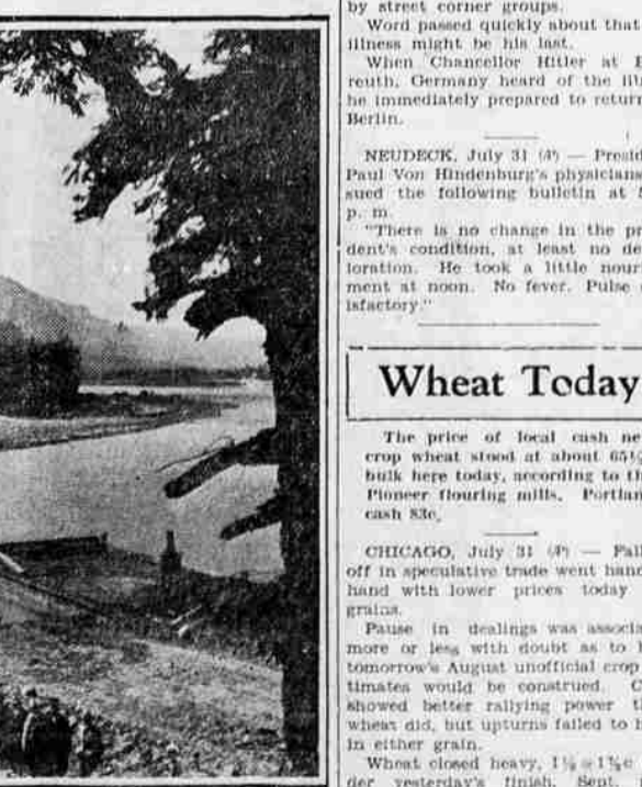
Cofferdams at the point between wooded mountains where a huge powerhouse will rise at Bonneville Dam... and begin putting to work one of the great rivers of the world. President Roosevelt will view this project (pictured above) when he visits Oregon this week.
