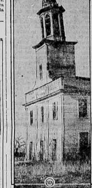
This is the Leaning Tower of Apollis, N. Y. Residents of the little village of 100 persons fear that the steeple may topple some day, pitching its 1300-pound bell through the roof of a nearby home. But nobody has offered to advance the money which would be required to have it taken down. The church has been practically abandoned for 40 years.
