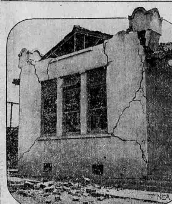
Here's what happened to a schoolhouse near Whittier, Cal., when a slight earthquake jolted the southern portion of the state the other day. No serious damage was done, but cracked walls, broken windows and loosened roofs gave citizens a number of thrills.
