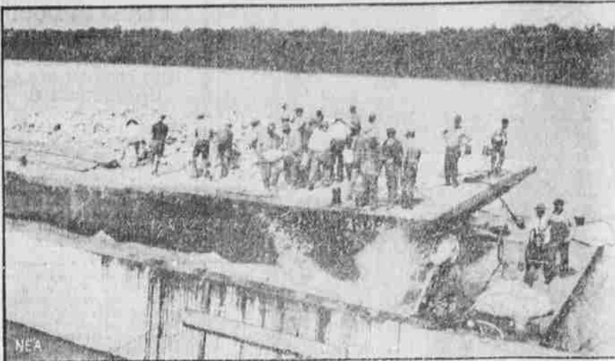
When a "sand boil" threatened the sea wall at Vicksburg, workmen and barges loaded with heavy rocks were rushed to the scene to avert a break in the wall. The sand boil caused when river water seeps under the wall gradually cutting a hole which makes it easy for the river to crack the weak sand wall. The rocks are thrown on the outside of the wall to choke the "boil" at its roots.
