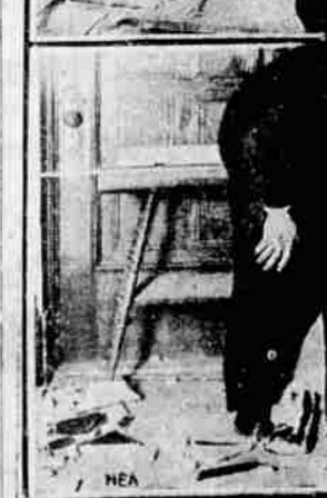
For the third time in a year bombers attacked the Church of Saints Peter and Paul, San Francisco, inflicting damage shown in the upper picture of the church entrance. Ironically, on the wall is the notice of $1000 reward for the bombers, posted after the second attack. Below is Father Oreste Trinchetti, parish rector, inspecting other damage.
