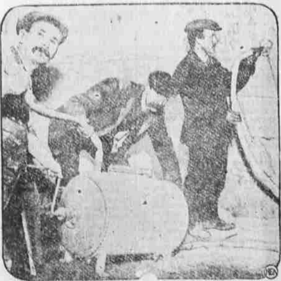
ST. PAUL'S CATHEDRAL, which has overlooked London for these hundreds of years, is crumbling with age. Workers are making desperate efforts to save it by filling the cracks with
