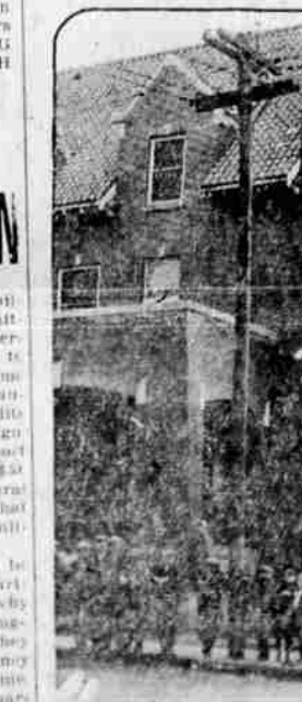
Citizens of Haleyville, Okla., were thrown into a panic when the Y. M. C. A. dropped three feet on its foundations into a tunnel of the abandoned Haleyville mine. The building is being saved by 1925.
