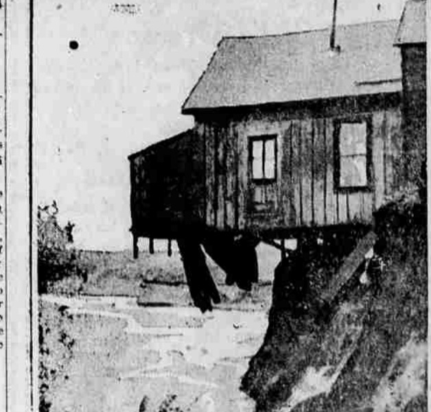
An example of the freakish activity of the waters that flooded Pueblo, Col. The kitchen of this house is hanging over the embankment without any support, except the long beams that reach out from the part of the house left on land.
