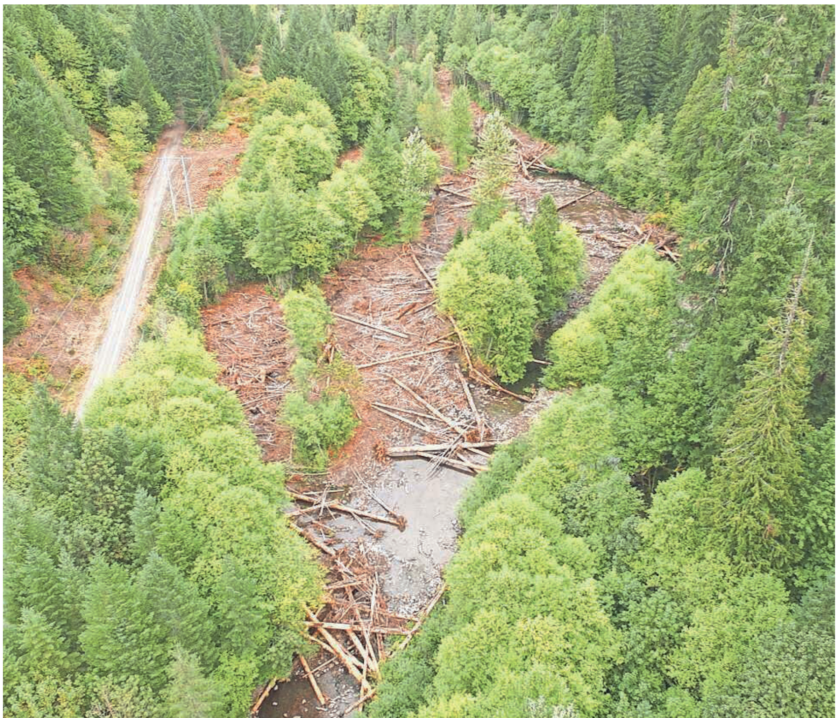
A floodplain restoration project has transformed a stretch of Deer Creek to be more hospitable to salmon spawning. A new phase of the project begins this summer. MCKENZIE WATERSHED COUNCIL
