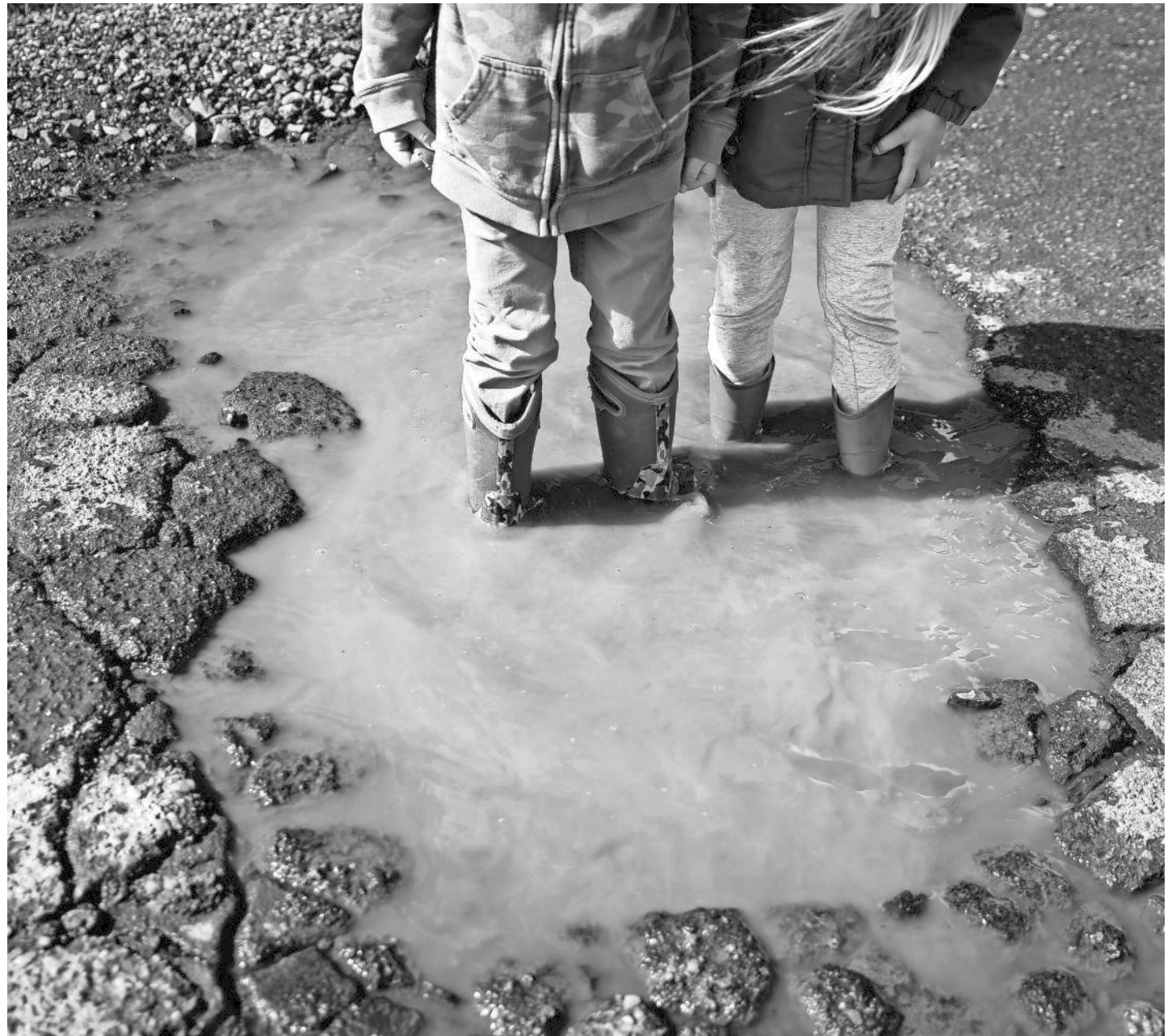
Matt Phipps' children stand in a pothole on Kenwood Avenue Northeast on March 9 in Salem.
