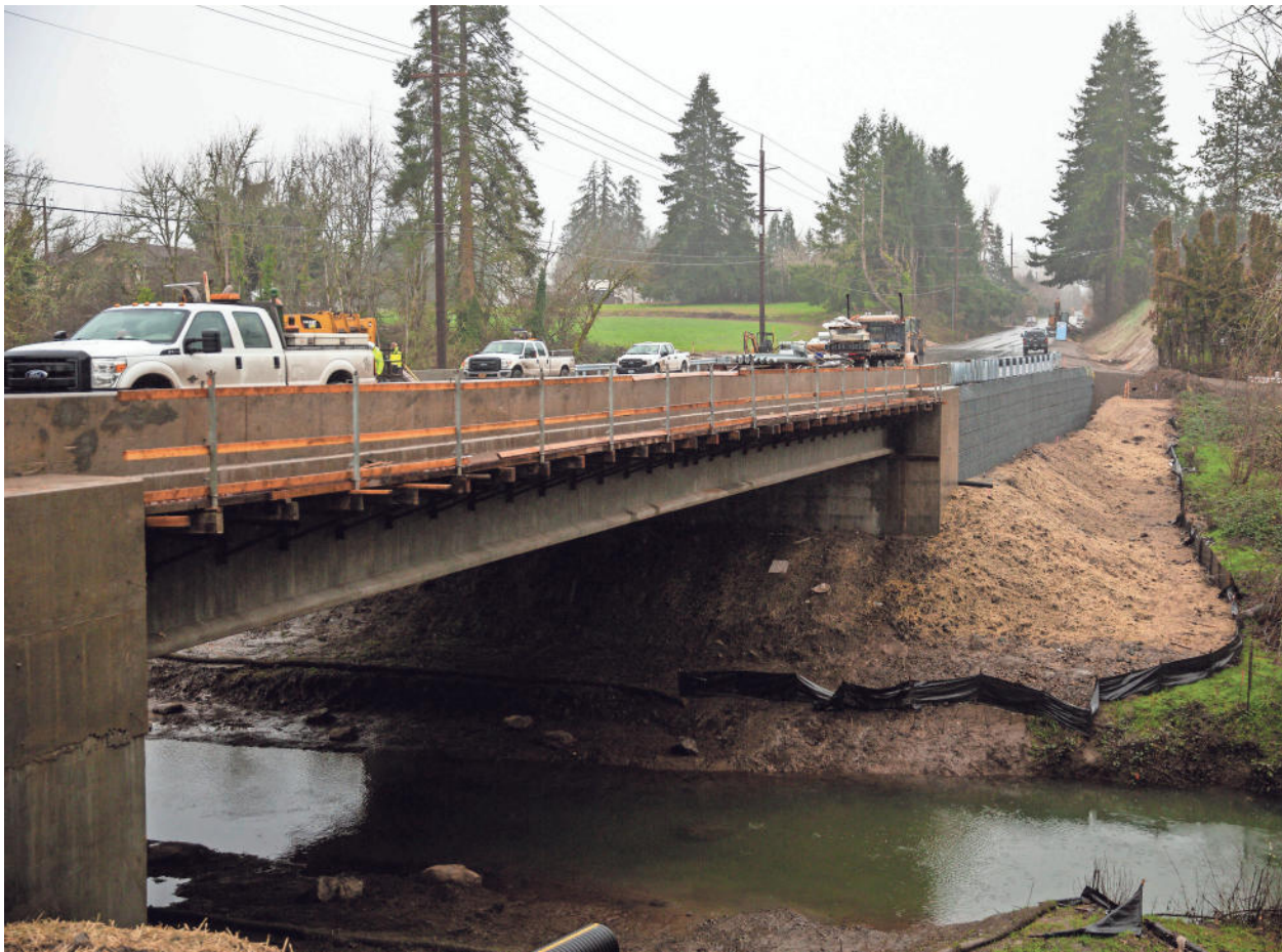
Construction work continues on the Silverton Road Northeast bridge over Little Pudding River in Salem.
