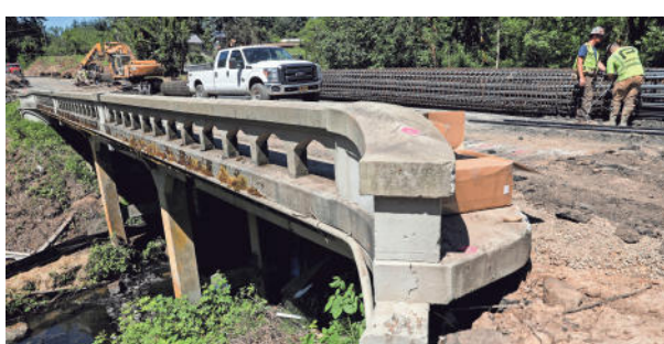
Crews work on a bridge replacement project on Silverton Road over the Little Pudding River in June. The bridge is now expected to reopen in late January. ABIGAIL DOLLINS / STATESMAN JOURNAL FILE
