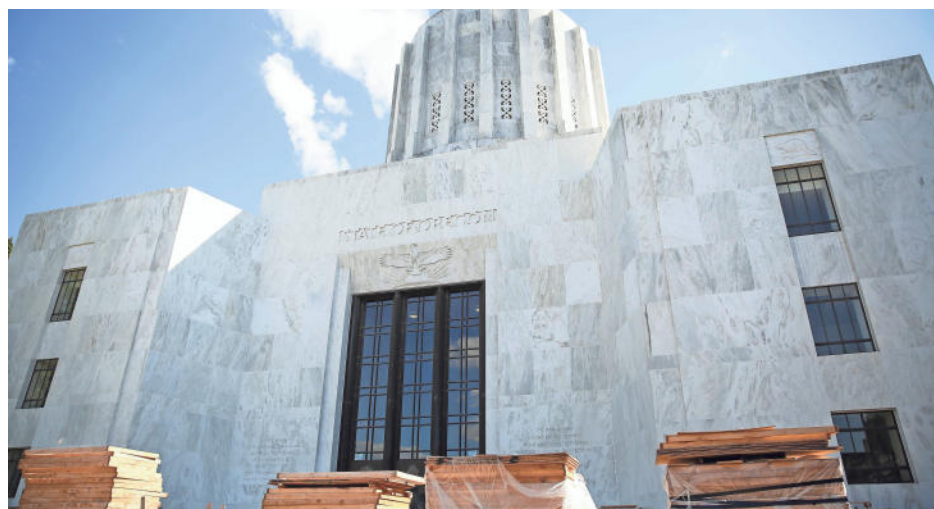
The front side of the Oregon State Capitol is under construction near Court Street Northeast on Wednesday, July 21, 2021 in Salem. ABIGAIL DOLLINS / STATESMAN JOURNAL
