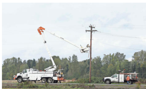
Portland General Electric crews finish repairing a power line near Faragate Street and Brown Island Road in south Salem on Sunday, Oct. 16, 2016, following a storm the night before. ANIELLE PETERSON / STATESMAN JOURNAL
