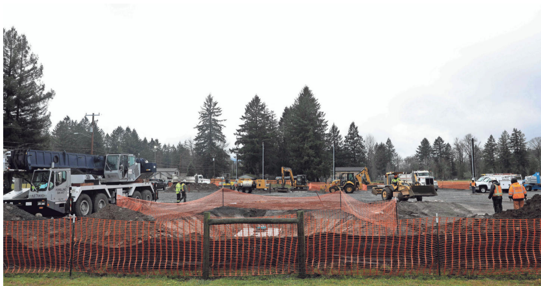
Crews from US West, Morello Construction and U.S. Army Corps of Engineers work to complete the first Santiam Canyon FEMA trailer site in Mill City.
