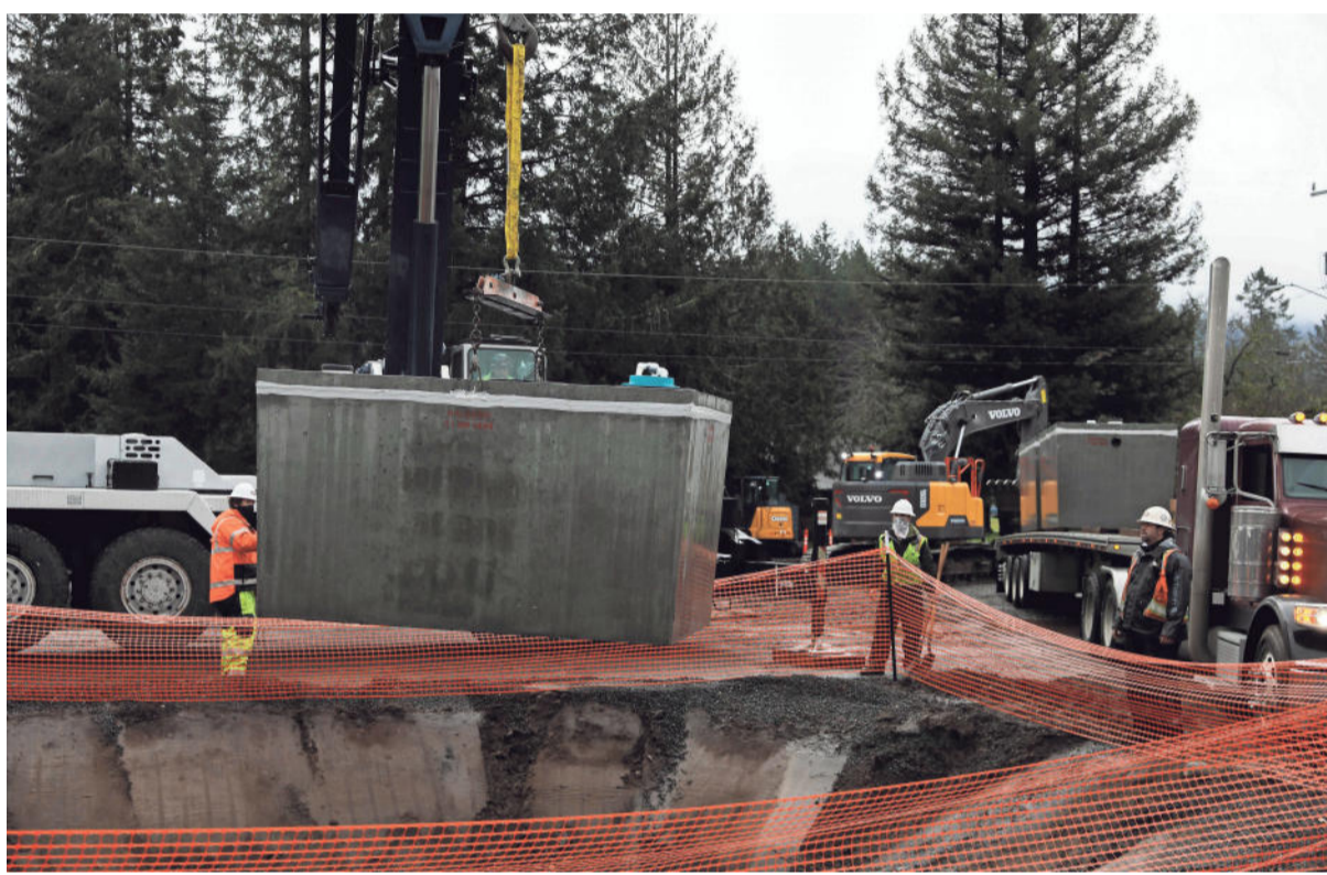
Construction crews lower a septic tank into the ground at the first Santiam Canyon temporary housing site organized by FEMA in Mill City. BRIAN HAYES / STATESMAN JOURNAL
