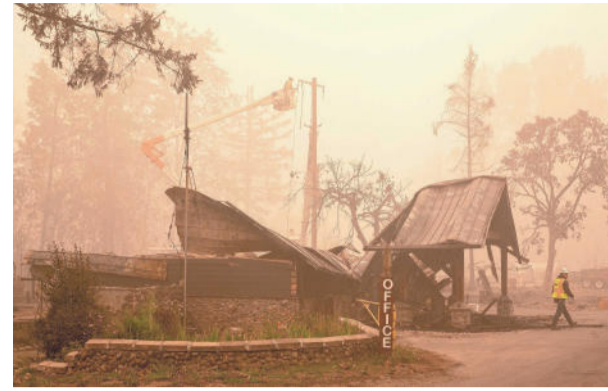
Workers continue to repair the power system after flames from the Beachie Creek Fire burned through Fishermen's Bend Recreation Site east of Salem. The wildfire caused the evacuation of 40,000 residents, killing four people and one is still missing. ROB SCHUMACHER/STATESMAN JOURNAL VIA USA TODAY NETWORK
