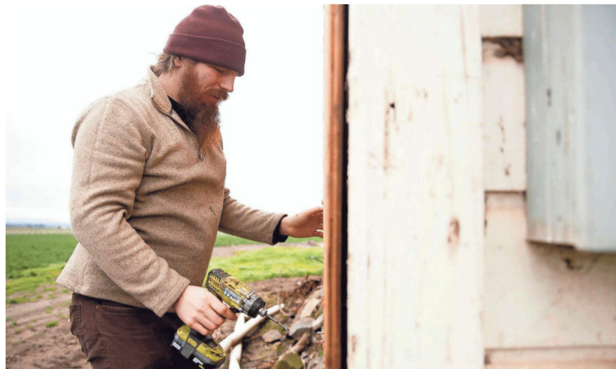
Nick Haas, of Portland, opens a doorway that was boarded up on a home built 1864 on a plot of land west of Silverton that was used in the Alan Alda movie "Isn't It Shocking?". The house has been uninhabited and dilapidated for years. Haas purchased the home in 2017 on the condition he move it to a new location and restore it. Photographed on Feb. 4, 2020. ANNA REED / STATESMAN JOURNAL
