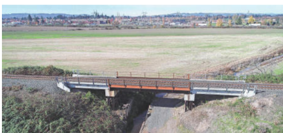
A newer railroad trestle crosses the area where a Southern Pacific passenger train plunged through a dilapidated trestle at Lake Labish on Nov. 12, 1890. DAVID DAVIS AND KELLY JORDAN / STATESMAN JOURNAL
