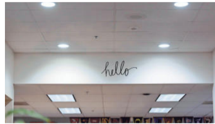
LED lights are installed in the counseling center at Silverton High School on Nov. 4, 2019. Bulbs and fixtures are being upgraded to LED lighting in the Silver Falls School District as part of a $1.8 million project. ANNA REED / STATESMAN JOURNAL
