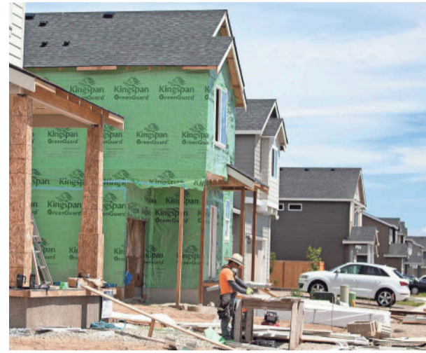
Apartments are built after a pesticide-contaminated soil cleanup on part of 150 acres in Northeast Salem on Friday. PHOTOS BY MICHAELA ROMÁN / STATESMAN JOURNAL
