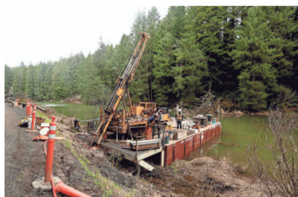
Crews work to drill and test soil samples for a proposed new dam at the Big Creek Reservoir near Newport. ANNA REED/STATESMAN JOURNAL
