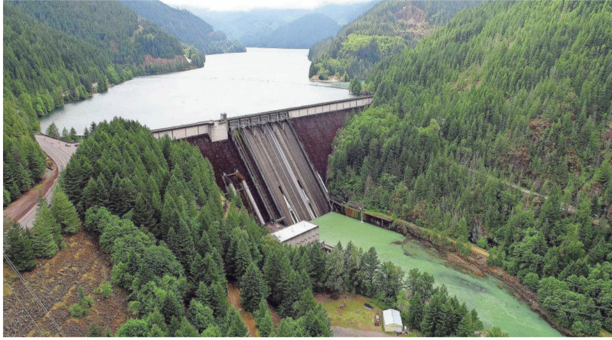
The Detroit Dam was built by the U.S. Army Corps of Engineers in the Willamette Valley and began operating in 1953. DAVID DAVIS AND KELLY JORDAN / STATESMAN JOURNAL
