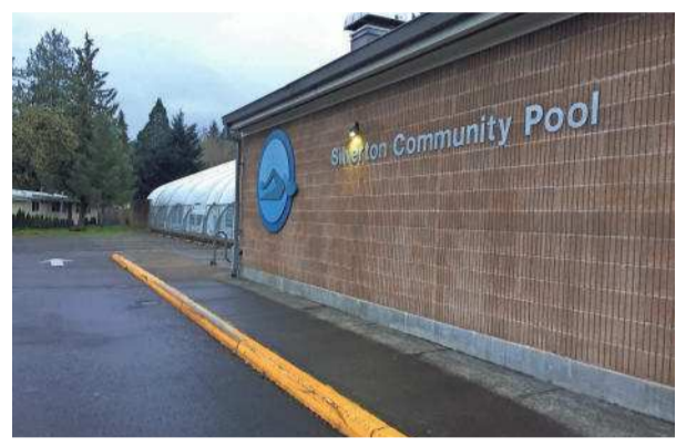
A 40-foot retaining wall has been recommended south of Silverton Community Pool. BILL POEHLER | STATESMAN JOURNAL
