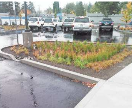
The rain garden infiltration system at the Starbucks on Commercial St SE is an example of the type of on-site stormwater retention projects that would be required of developers in smaller cities under the new permit. IMAGE PROVIDED BY THE CITY OF SALEM
