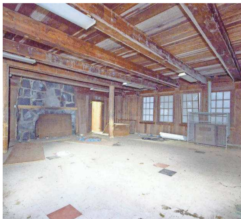
Dwight and Susan Sheets are seeking other grants and fundraising to cover the potential $2 million to $3 million needed to fully restore the ski lodge, which sits on 26 acres near the top of Santiam Pass.
