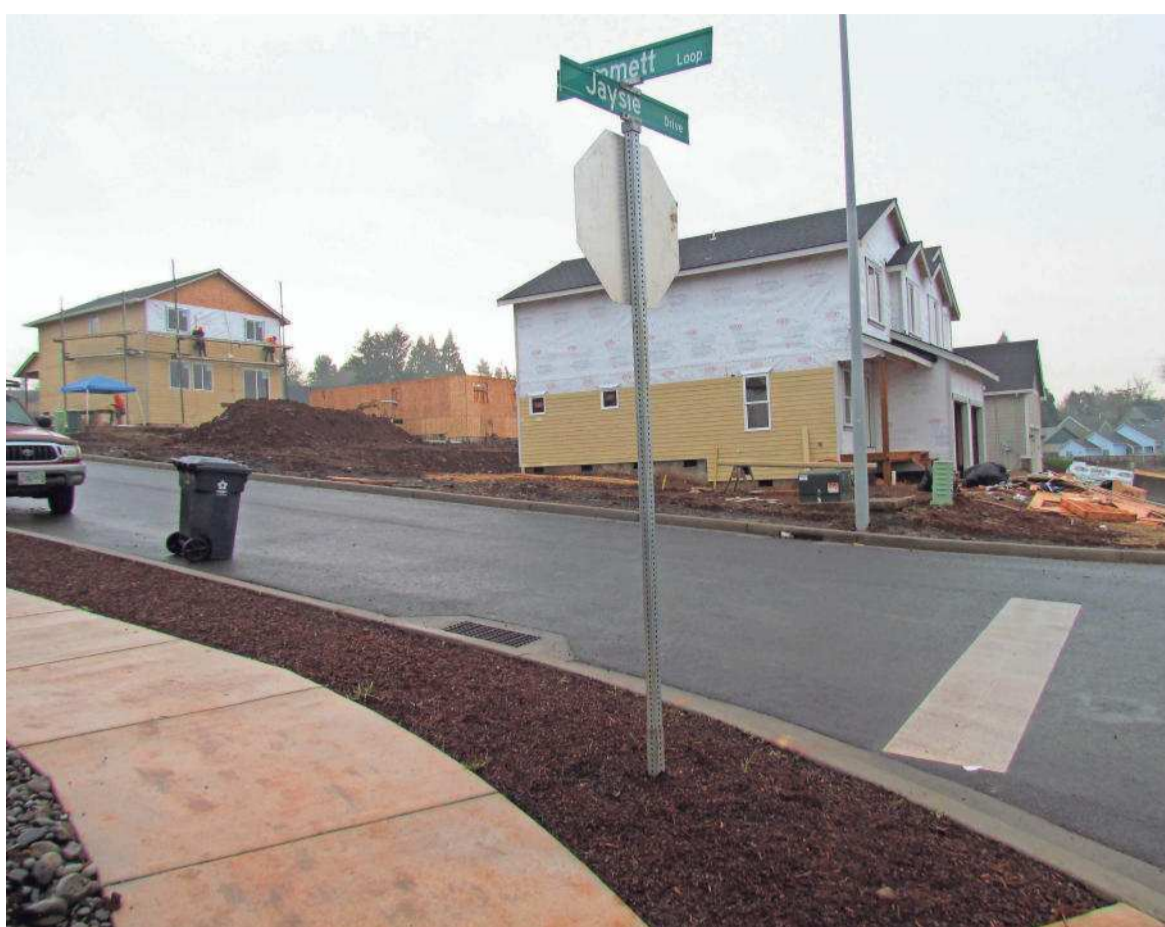
New homes under construction in Silverton at a recent subdivision on Jaysie Drive located off of Steelhammer Road. JUSTIN MUCH | SILVERTON APPEAL TRIBUNE
