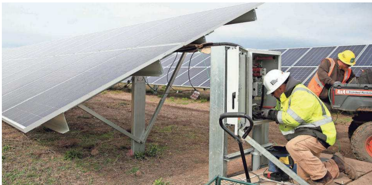
Electricians Ryan Lichty, left, of Silverton, and David Hammang, of Dayton, work on the Cypress Creek Renewables solar energy farm near Silverton on Oct. 17. ANNA REED / STATESMAN JOURNAL
