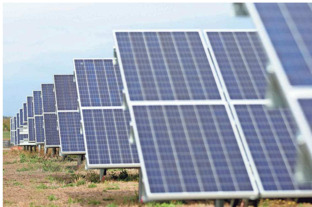
The Cypress Creek Renewables solar energy farm is seen under construction near Silverton on Oct. 17. Five new solar farms are planned to be built in Marion and Polk counties. ANNA REED/STATESMAN JOURNAL
