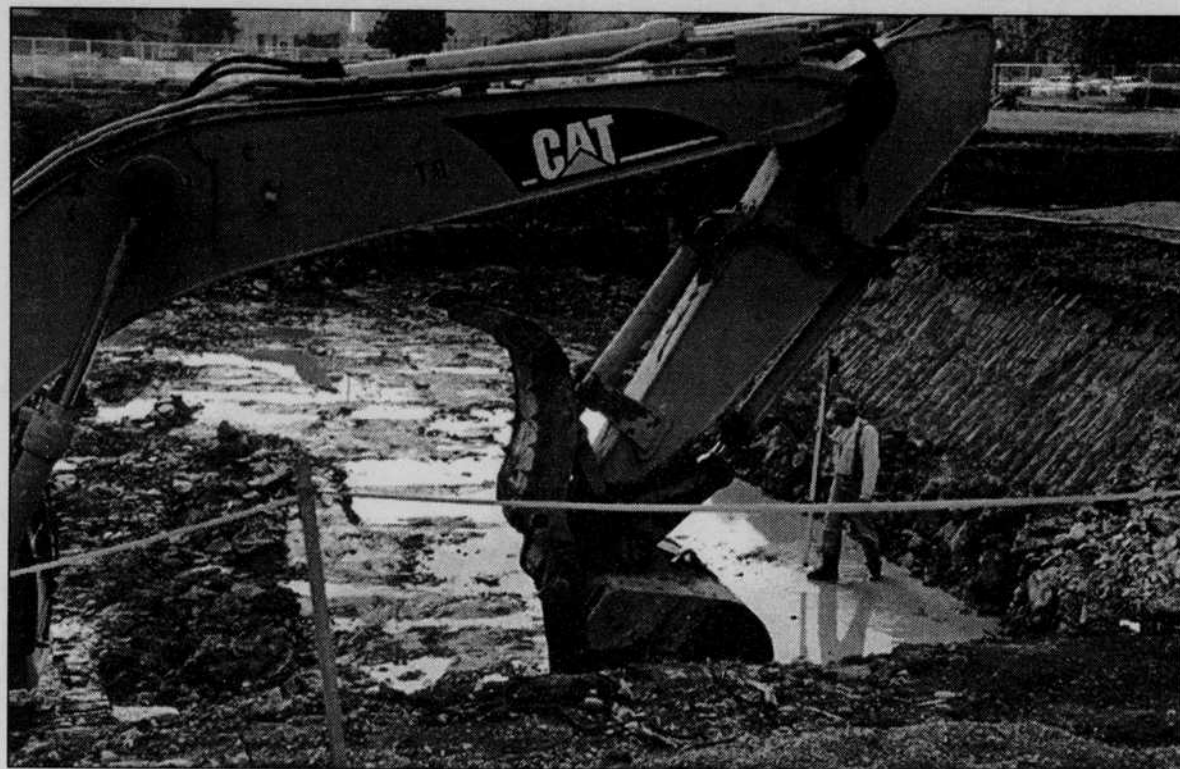
John Gardner of Delta Sand and Gravel works Tuesday on the construction of The Living Learning Center, which is being built next to the Walton Complex.
