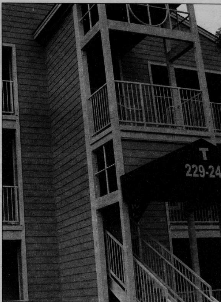
Places like the University Commons are furnished apartment complexes built for students and include access to a pool, fitness center and more. Emerald
