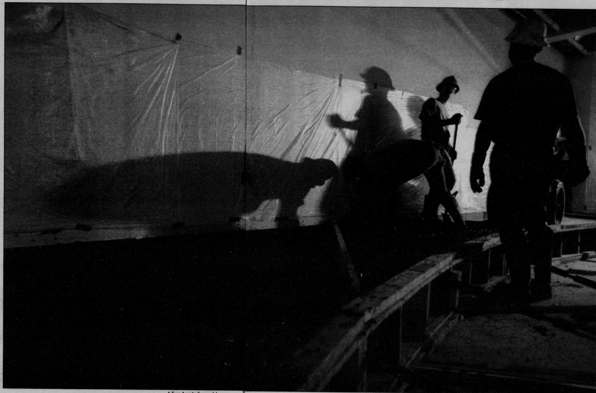
Adam Amato Emerald (Above) Concrete finishers smooth out the upper level of one of the raised seating classrooms on the third floor of the Lillis Business Complex.
