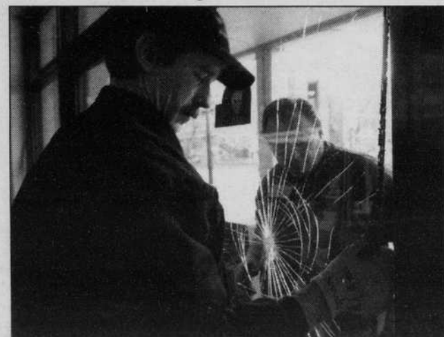
Bob Seymour (left) and Tom Boren from Lane County Glass repair a broken window at the University Bookstore Wednesday morning after it was hit by vandalism. Adam Amato Emerald
